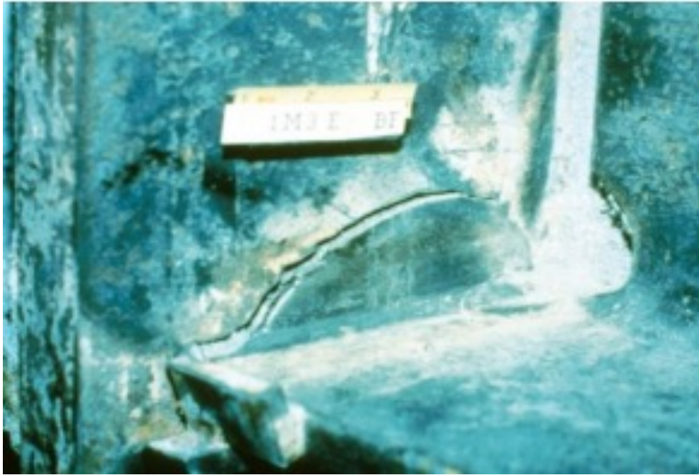
The 1994 Northridge (California, USA) earthquake
