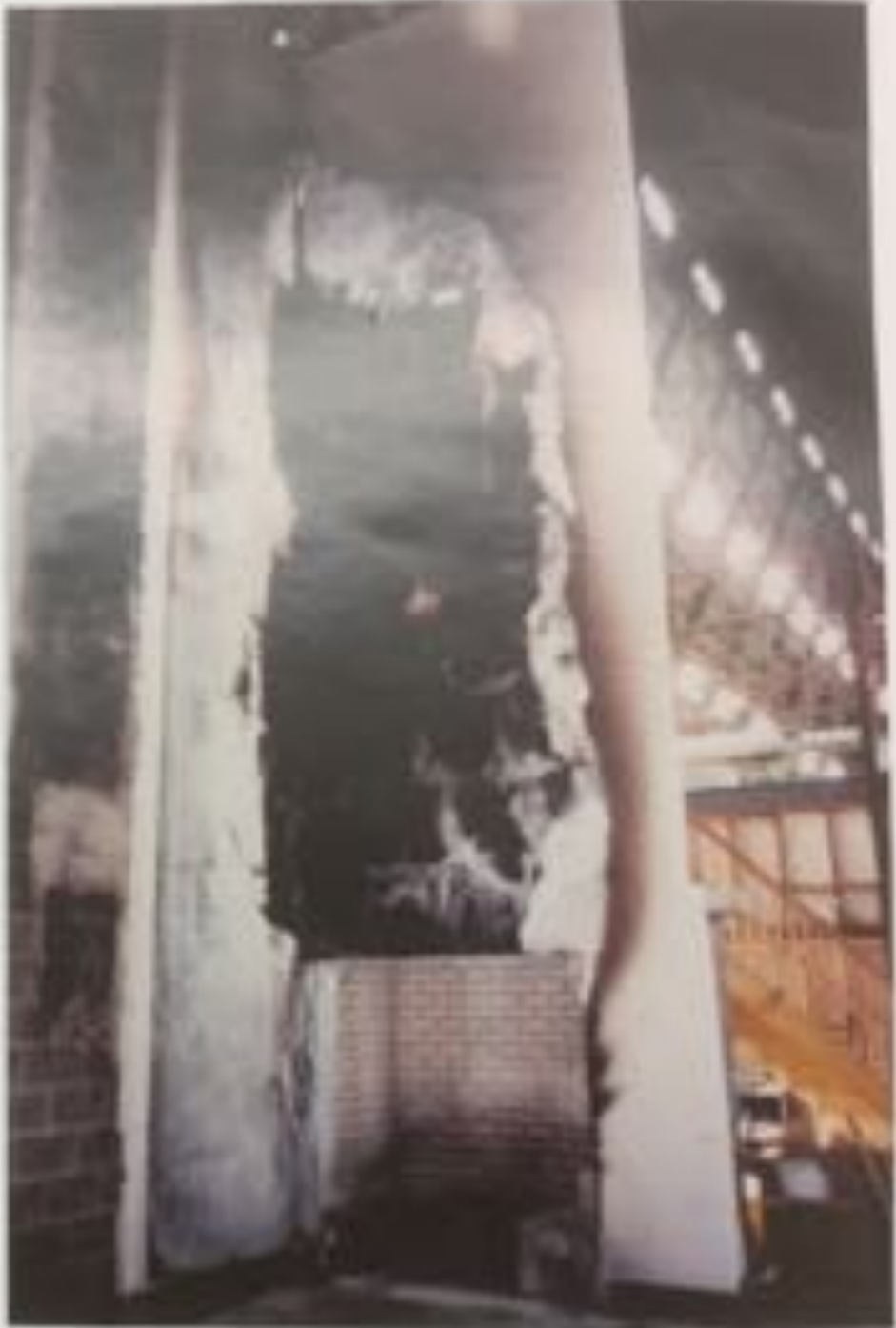
Figure 10: Thermosetting core without adequate frings or fire breaks
