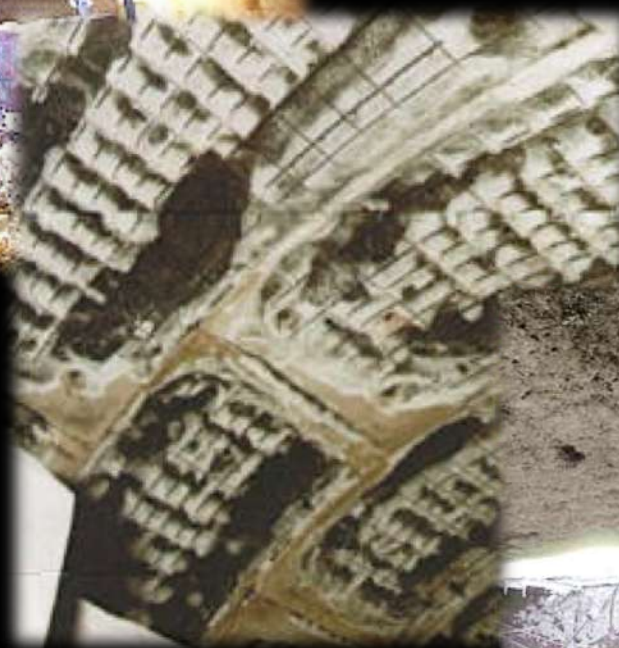
Channel Tunnel fire Source: www.phys.tue.nl/
