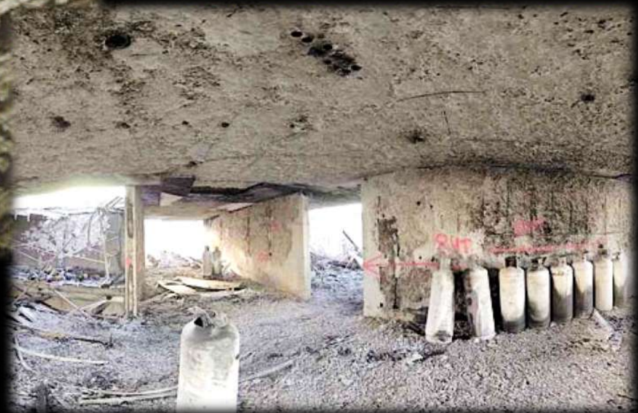
Spalling of a building under construction Source: www.panoramafactory.net
