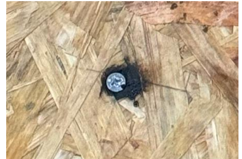
Local charring of timber around a metal shear connector
