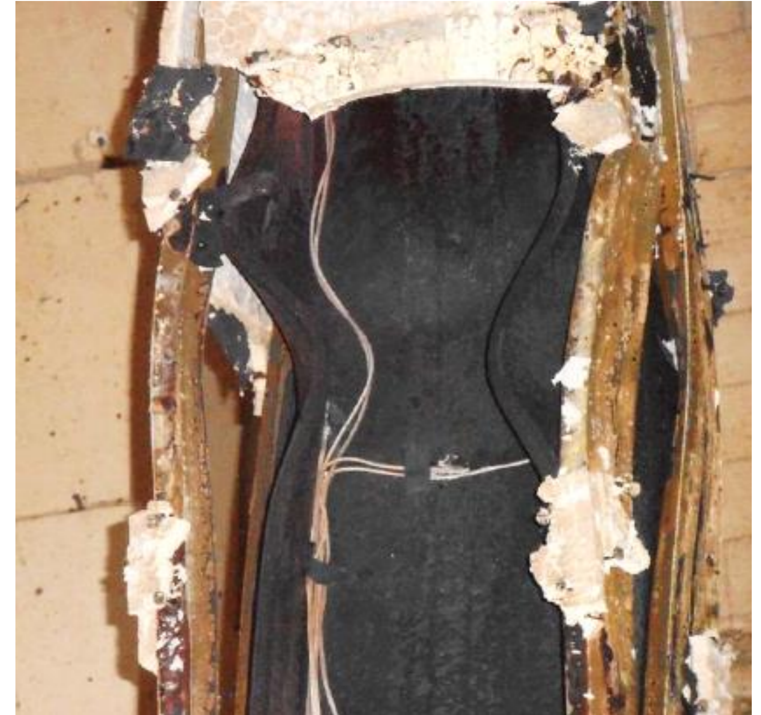
Local buckling failure of the steel column – Sample 120B
